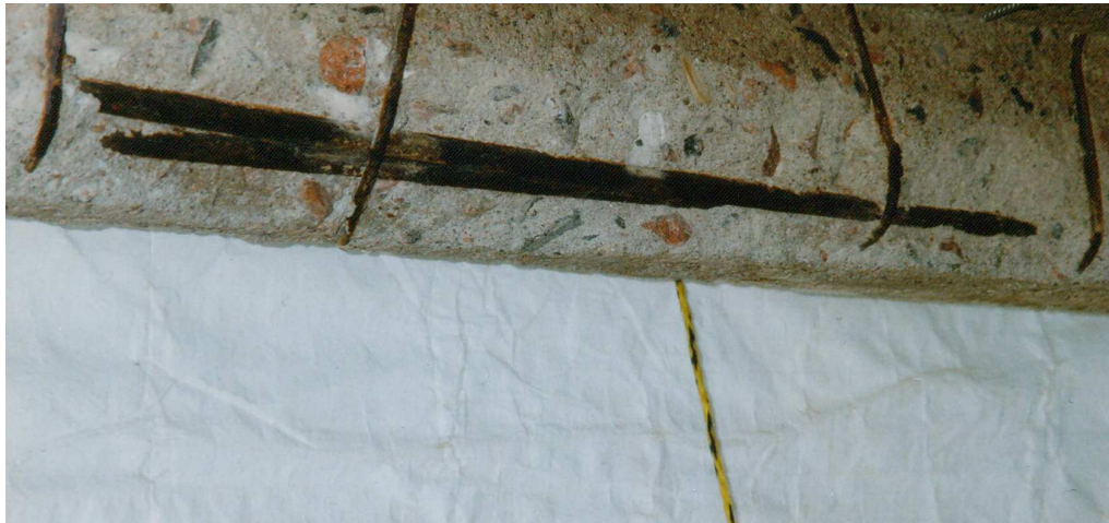
Photograph 5. Rand beam of the roof. Old bars visible.
